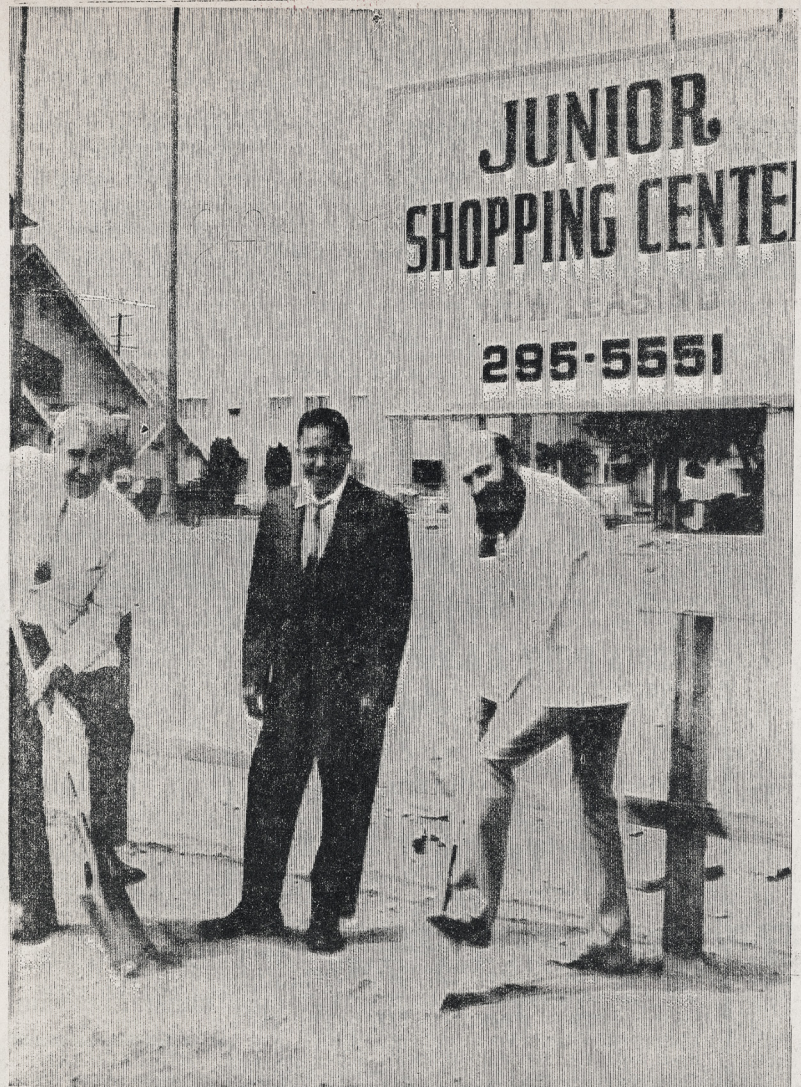
GROUND-BREAKING: Participating in ground-breaking ceremony for the new "Campus Center" are, left to right, Jaimie Monroy, CRA Hoover Project Manager; Vincent Proby, project architect; and Jerry J. Bloom, president of Bloom Development Co., Inc.
